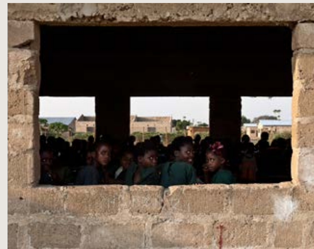
Pupils at Nakambala Basic School, next to the Zambia Sugar estate, in their unfinished classroom.
